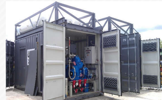
Gas Generation & Distribution
