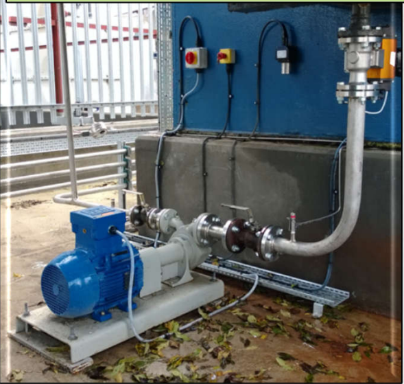
Pump Systems (Clean Agent)
