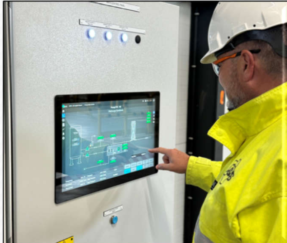
Central PLC & E/Stop Hub (HMI optional)
