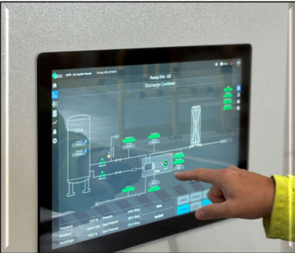
Pump Panel HMI
