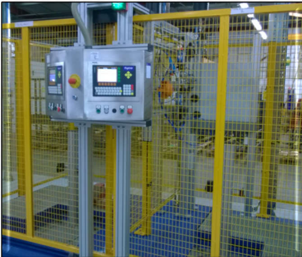
Operator Interface (CA) (HMI)
