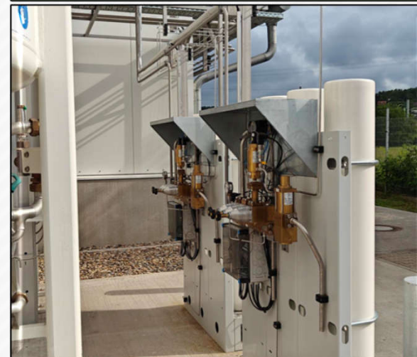
Skid & 3 Cylinder Buffer
