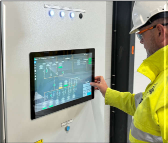
Central PLC & E/Stop Hub
